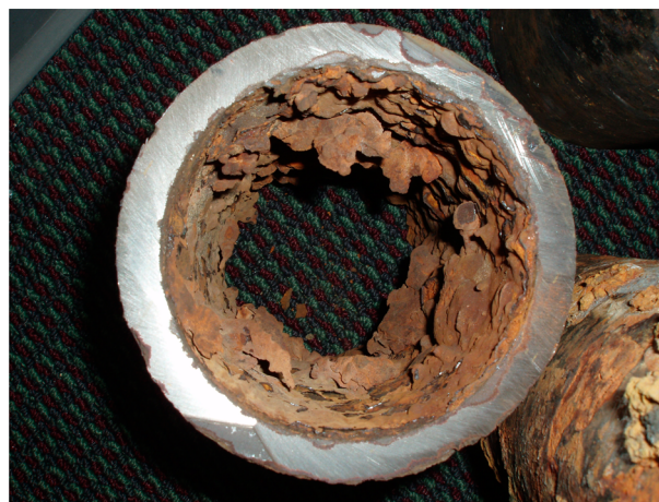
Figure 1. Pipe scale from a ductile iron water main in Iowa. Note the iron-containing nodules that have formed on the inside of the pipe, which could dissolve or break away in the presence of corrosive water. Photo credit: Richard L. Valentine; used with permission.
