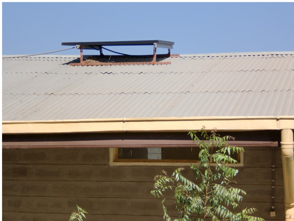
Fig. 3. PV panel installed on a health station's roof.
