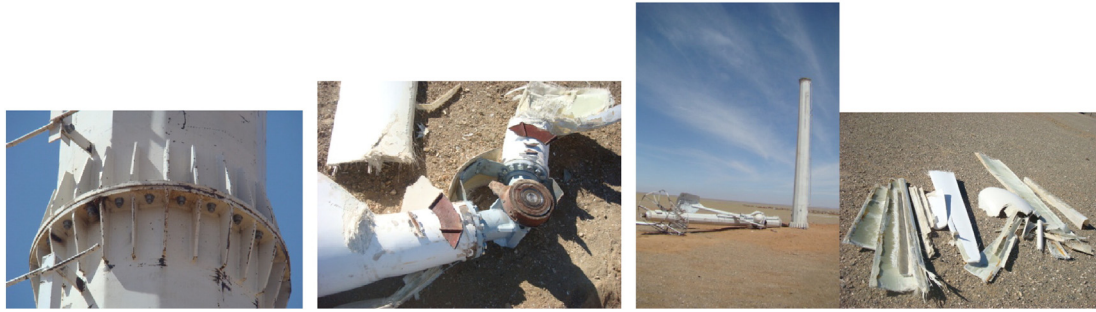
Fig. 3. A view of broken wind turbine (Turbine #2 Bogd soum).
