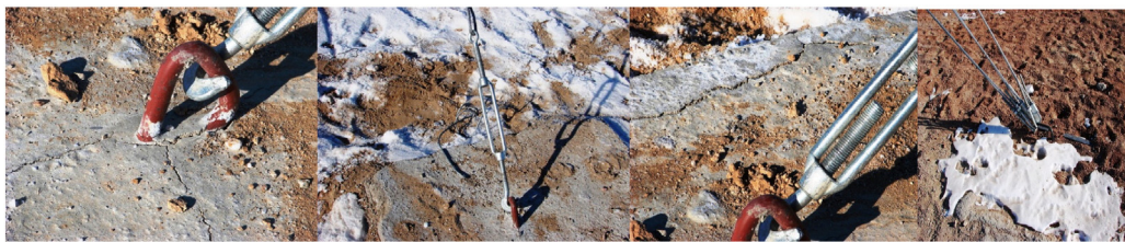
Fig. 4. Structural damage on wire-fixing foundation (Khatanbulag soum).
