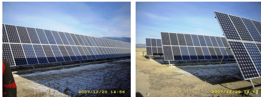
Fig. 7. View of the incorrectly installed solar PV arrays (Tsetseg soum , 2009).
